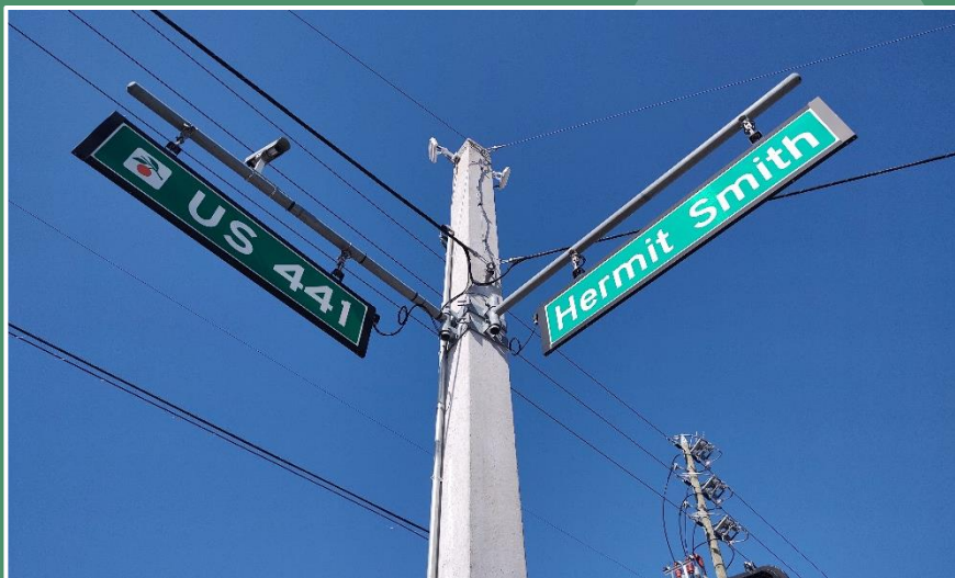
Two (2) microwave radar sensors installed directly to the concrete strain pole. (Orange County)
