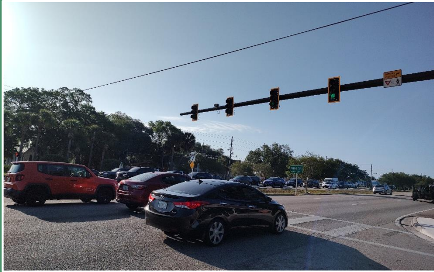
Hybrid radar-video unit installed on mast arm on the far-side of signalized intersection approach. (Osceola County)
