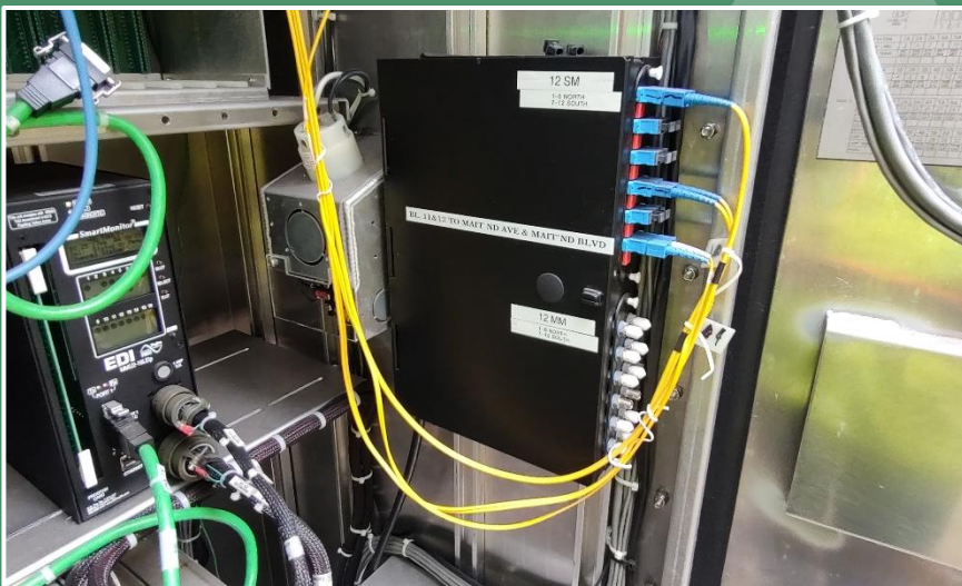
Fiber optic patch panel installed in controller cabinet assembly with two (2) fully terminated twelve-count connector panels. (City of Orlando)
