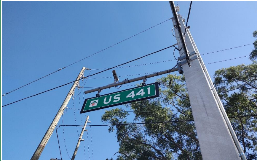
Video detection camera installed on cantilevered mounting arm for span wire intersection. (Orange County)
