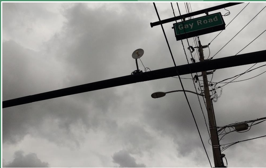
Dish-style point-to-point wireless radio installed on mast arm structure. (City of Orlando)
