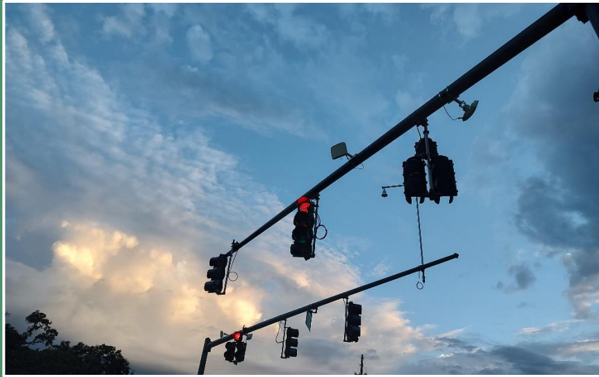
Multiple microwave radar sensors installed on mast arm assemblies on the near side of the intersection for stop bar detection. ( Volusia County )
