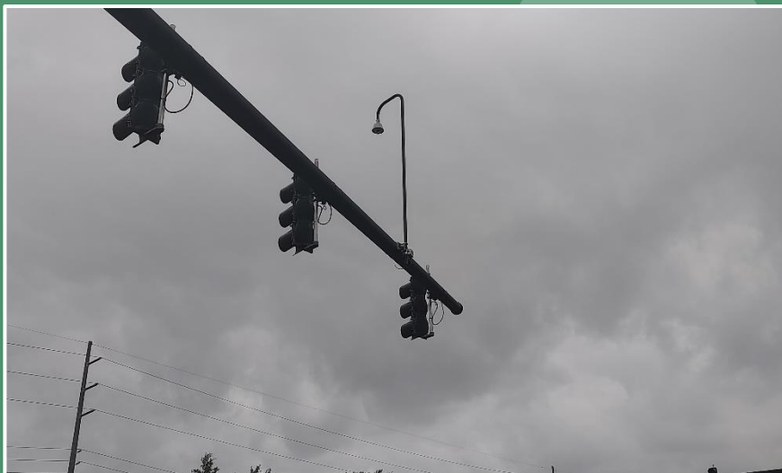
Mast arm structure with omnidirectional camera sensor positioned towards the center of the signalized intersection. (Seminole County)
