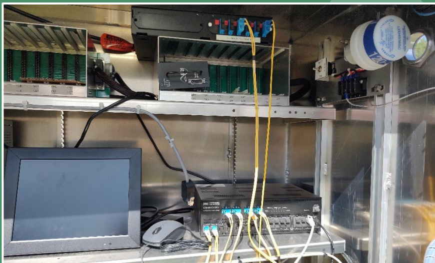
Connections between the fiber optic patch panel and the managed field Ethernet switch is developed using fiber optic jumpers; yellow for single-mode, orange for multi-mode. (Lake County)
