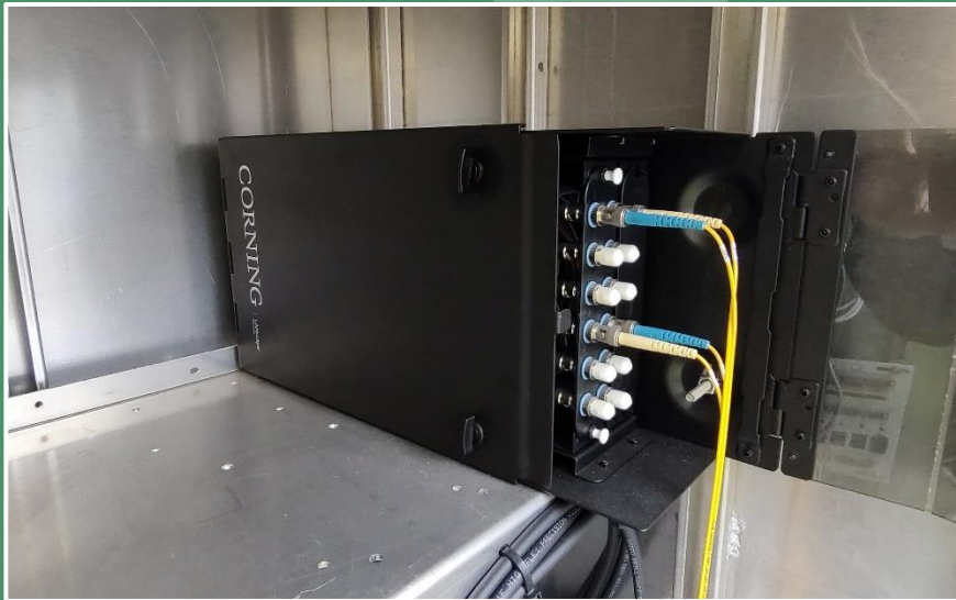
Shelf-mounted fiber optic patch panel with twelve-count connector panel. (City of Orlando)
