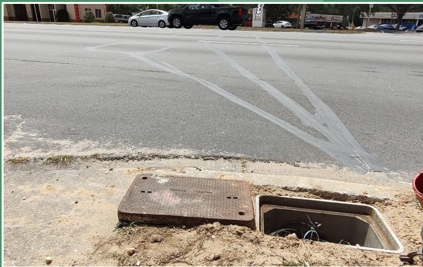
Loop lead-in wires for advanced detection cut in asphalt pavement surface to homerun pull box. (Marion County)
