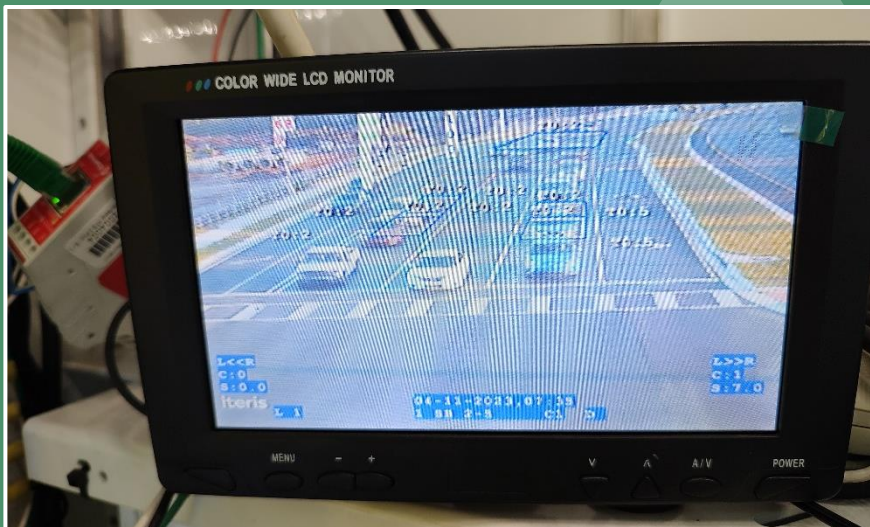
LCD color monitor installed in controller cabinet assembly displaying active vehicle calls for advanced detection zones. (Orange County)
