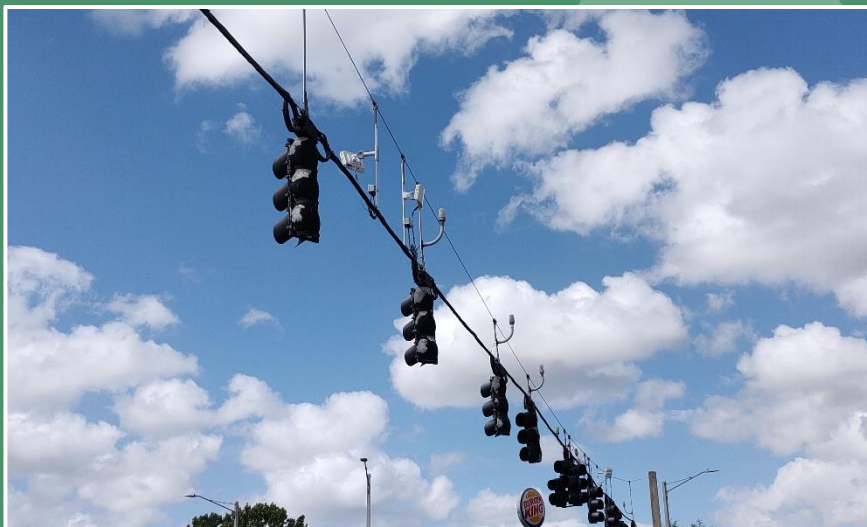
Multiple microwave radar sensors installed for span wire intersection stop bar detection. ( Lake County )
