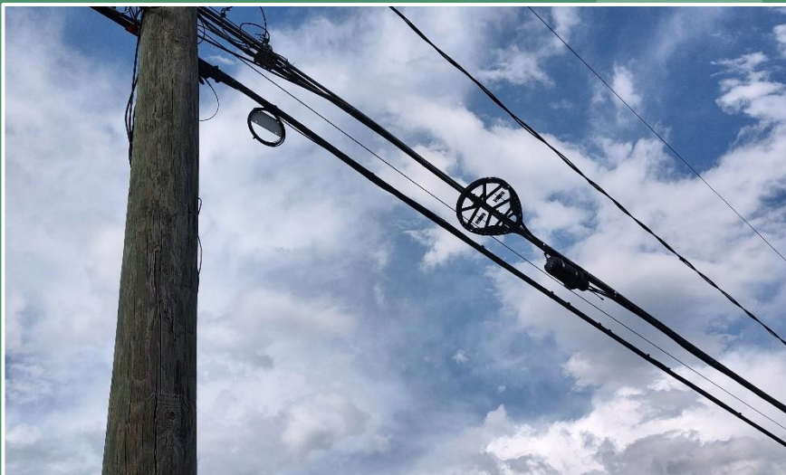
Example aerial fiber optic line with snowshoe cable storage fixture and overhead splice enclosure. (City of Orlando)
