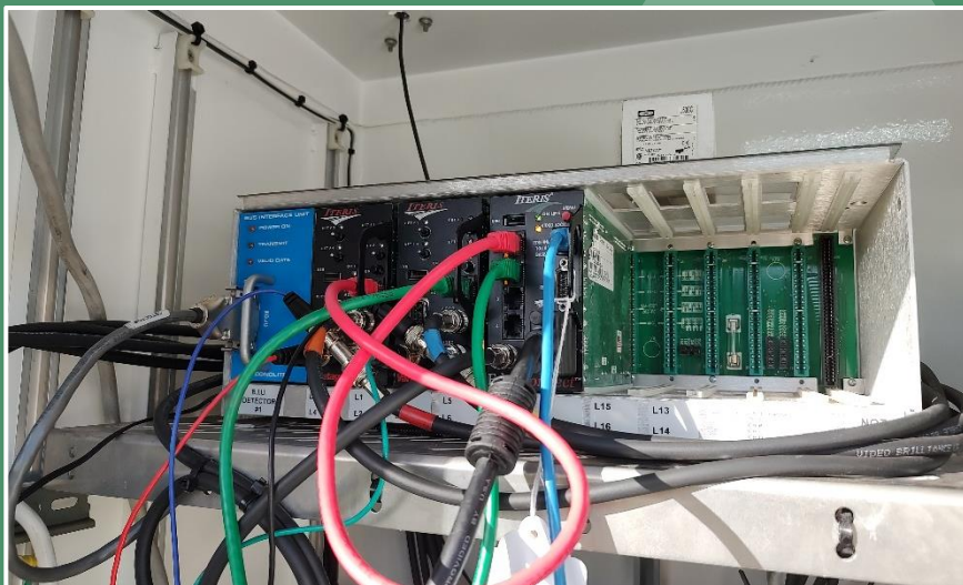
Image processing cards for video vehicle detection system installed in detector rack with bus interface unit (BIU) in controller cabinet assembly. (Osceola County)
