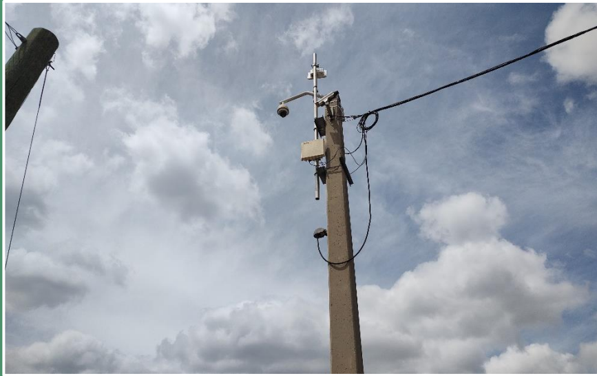
Multiple point-to-point wireless radios installed to vertical riser mounting arm creating connection between signalized intersections. (Marion County)
