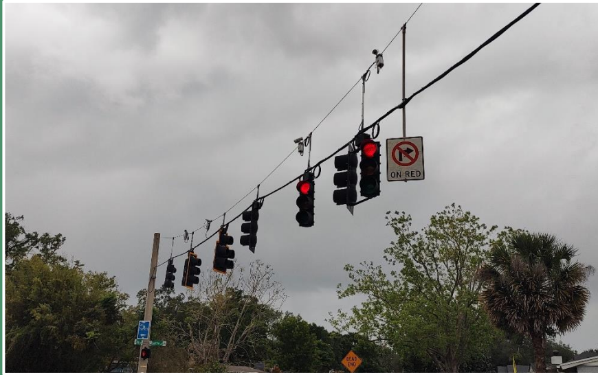
Video detection cameras installed directly to the catenary wire of a span wire intersection. (City of Orlando)
