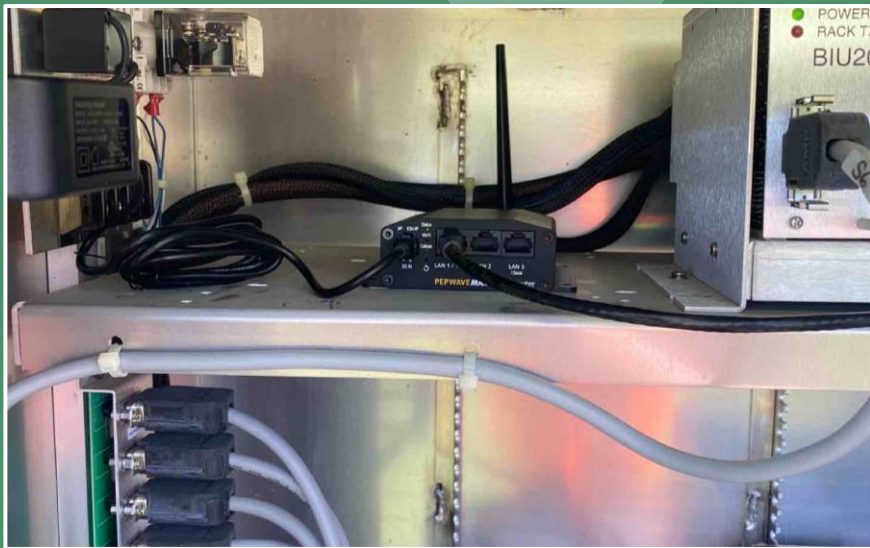
Cellular modem with embedded antenna; however, external antennas may be installed to the exterior of controller cabinet assemblies to boost signal strength, where needed. (Marion County)
