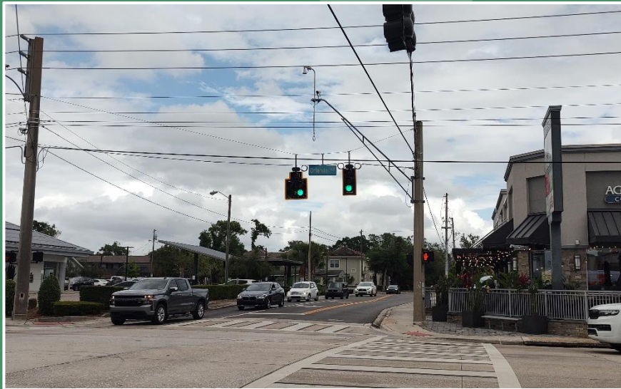
Video detection camera mounted on luminaire support arm for increased elevation above the road surface in a span wire intersection. (City of Orlando)
