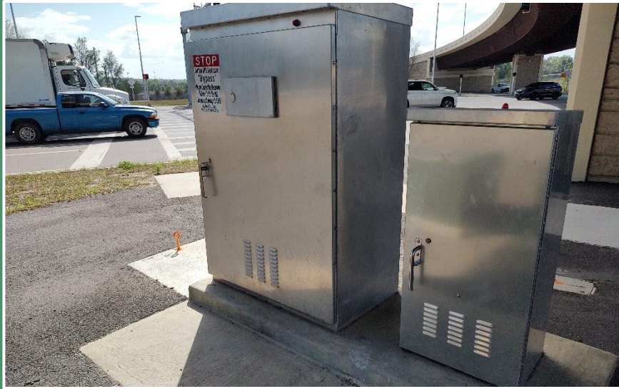
NEMA Type 6 controller cabinet assembly with stand-alone UPS cabinet on shared concrete base (foundation) with generator security anchor. (Lake County)
