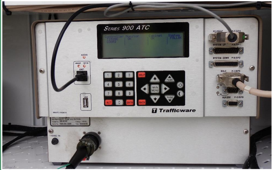
Trafficware (now Cubic ITS) 980-ATC unit, NEMA TS-2, Type 1 model. (Seminole County)
