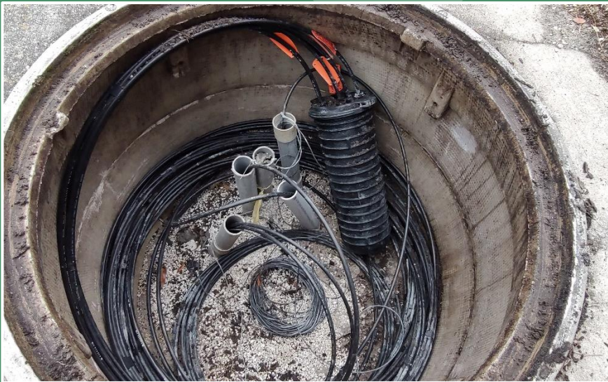
Interior of round fiber optic splice vault with conduit sweeps, cabling slack, and underground splice enclosure. (Orange County)
