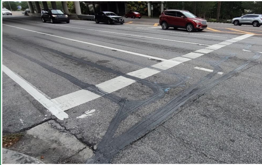
Type F inductive loops installed forty feet (40') in length with loop lead-in cuts. (City of Maitland)
