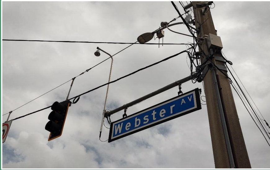
Omni-directional camera sensor installed on cantilevered mounting arm for span wire intersection. (City of Orlando)
