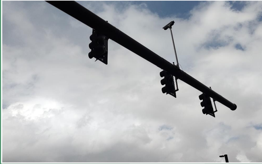
Vertical riser mounting arm installed to provide greater elevation of video detection camera above the roadway surface for advanced detection zones. (City of Orlando)
