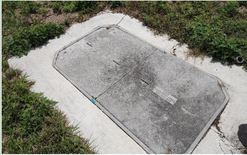
Two-section lid fiber optic splice vault (30" X 60") with concrete apron. (Marion County)
