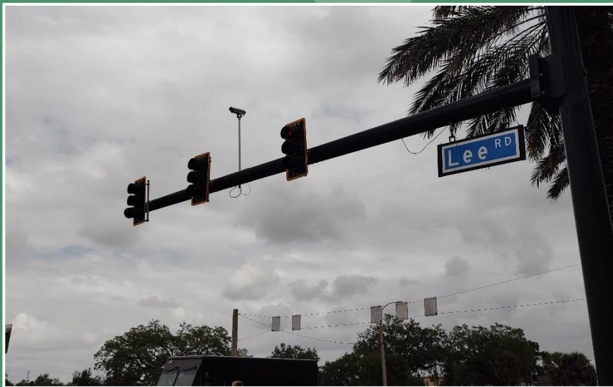
Mast arm structure with video detection camera on vertical riser mounting arm. (City of Orlando)
