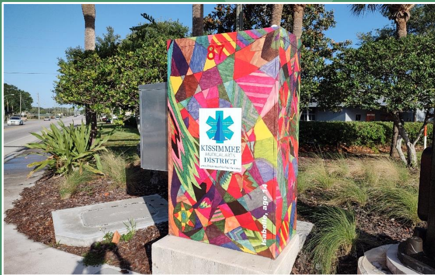
“Piggyback” UPS cabinet attached to the exterior side wall of the NEMA Type 6 controller cabinet assembly; some agencies may elect to wrap cabinet exteriors to match local aesthetic requirements. (Osceola County)
