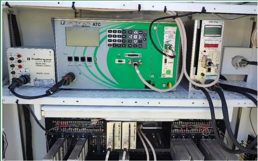
Trafficware (now Cubic ITS) ATC unit, NEMA TS-2, Type 1 model. (Brevard County)
