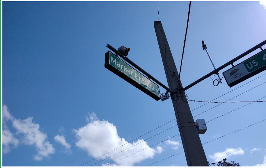
Hybrid video-radar unit installed on cantilevered mounting arm attached to the concrete strain pole at a span wire intersection. ( Lake County )
