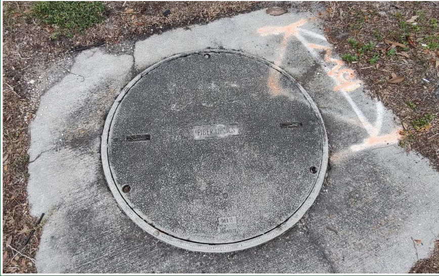
Typical round fiber optic splice vault (36" diameter) installed at the base of the controller cabinet assembly. (City of Orlando)
