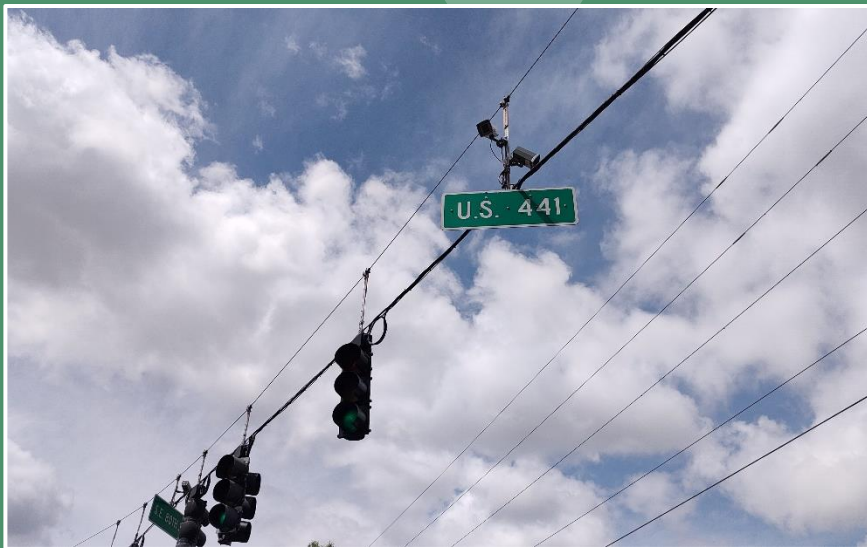
Span wire intersection with microwave radar sensors installed using mounting assembly attached to the catenary and messenger wires. ( Marion County )
